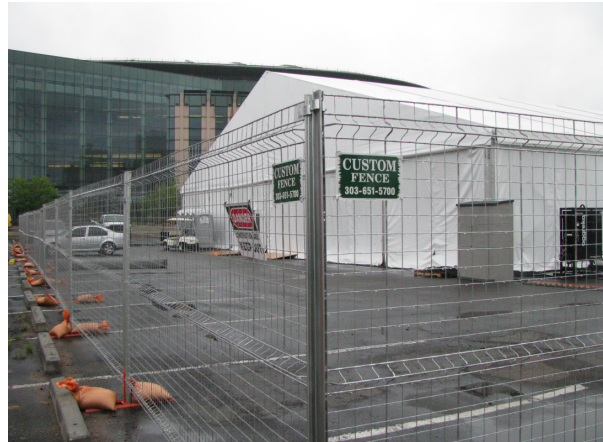
Media tents set up outside the Pepsi Center in Denver were secured by V-Squared Temporary fence provided by Custom Fence Supply.
